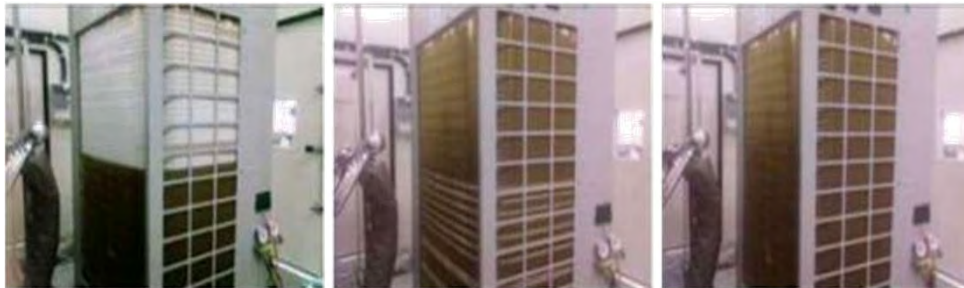
1. Lower HEX Defrost 2. Upper HEX Defrost 3. Lower HEX Defrost
