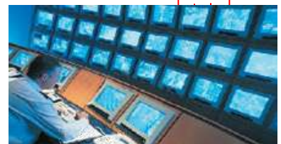
BMS (Building management system)
