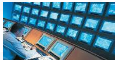
BMS (Building management system)
